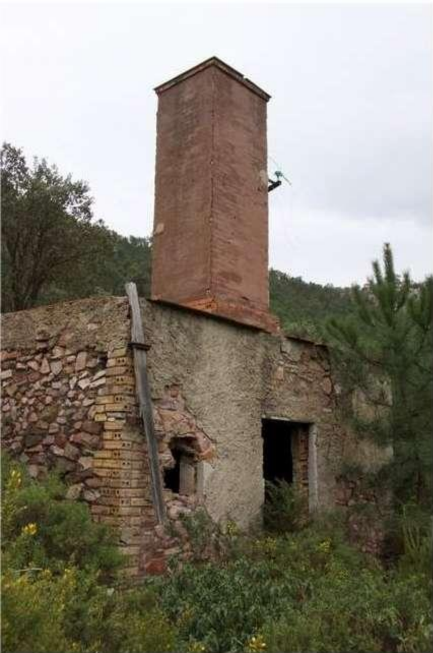
Trafo (Fot. J.M. Sanchis, 2009)
